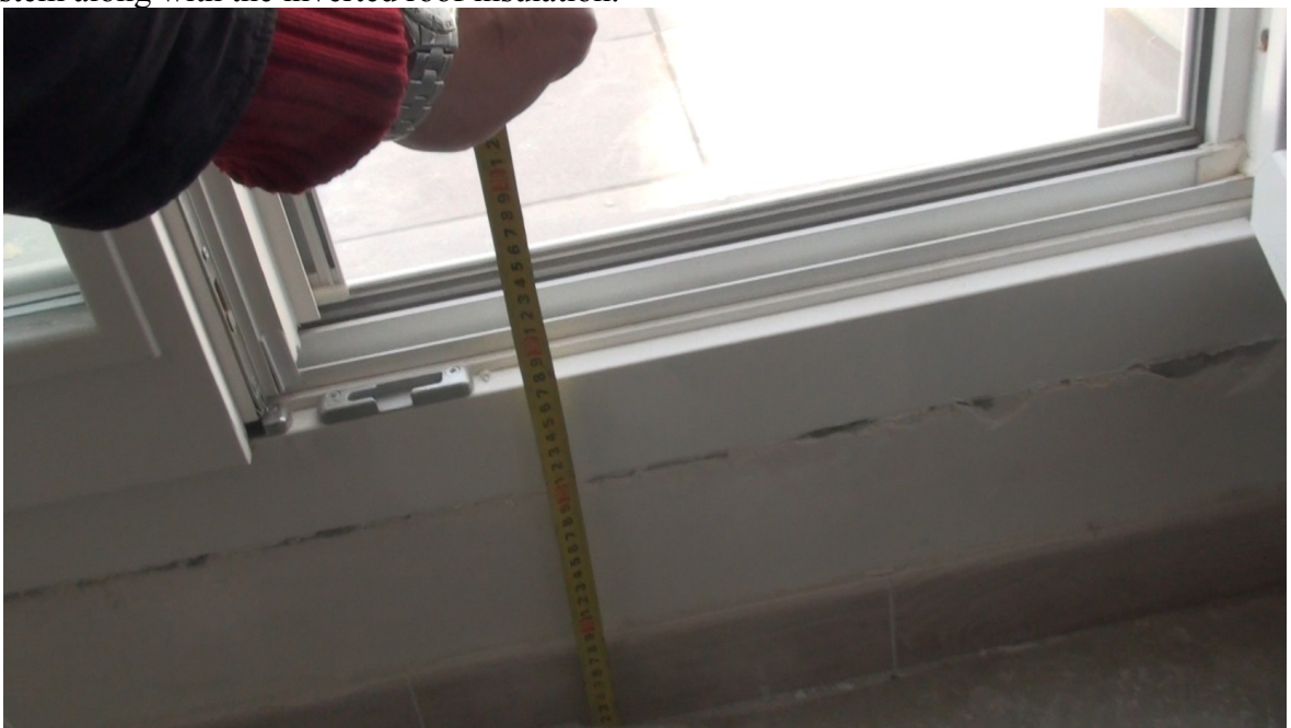
Difference in height of the floor of the door due to the insulation of the roof in the last floor
