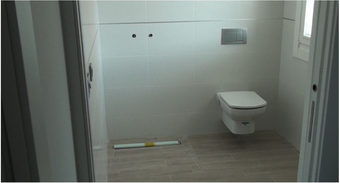
Toilet with sink shower in the master bedroom floor
