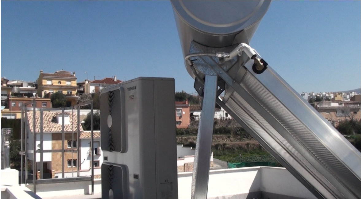
Installation on the roof above the flat roof of the tower of the last storey
