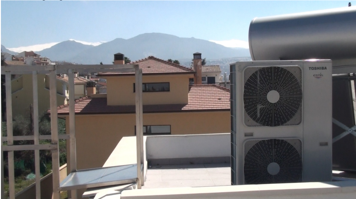
Exterior unit of heat pump of system Estia
