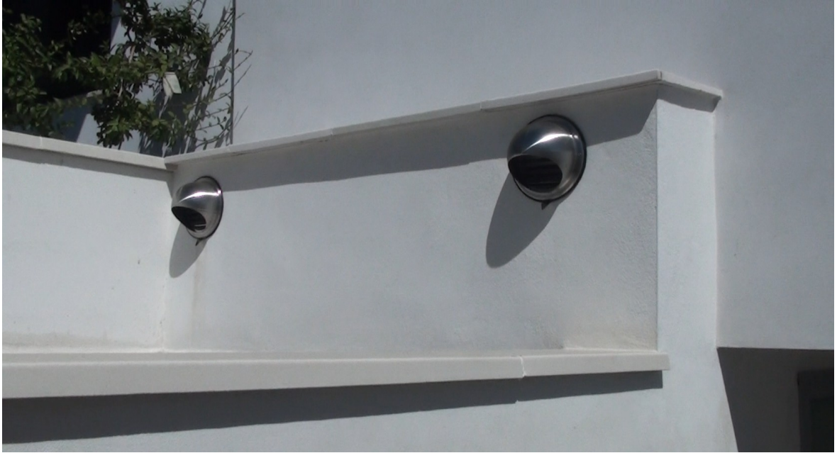
Taking clean air from outside of home and ventilation of the basement
