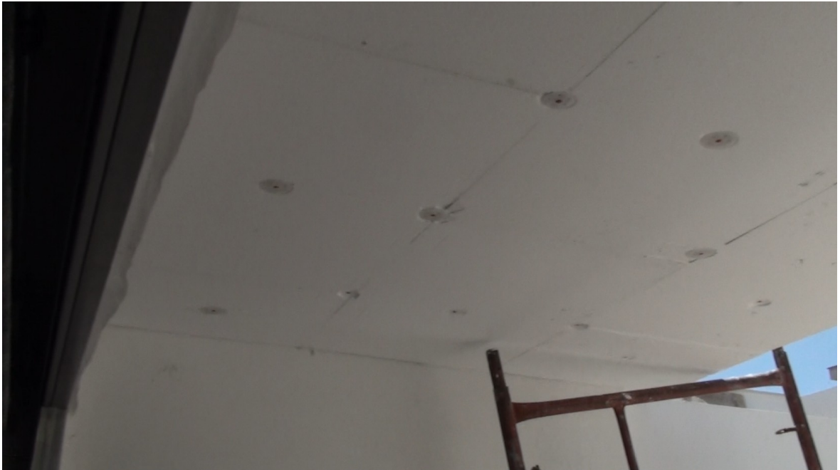
EPS insulation boards of 5 cm fixed to the ceiling of the garage door
