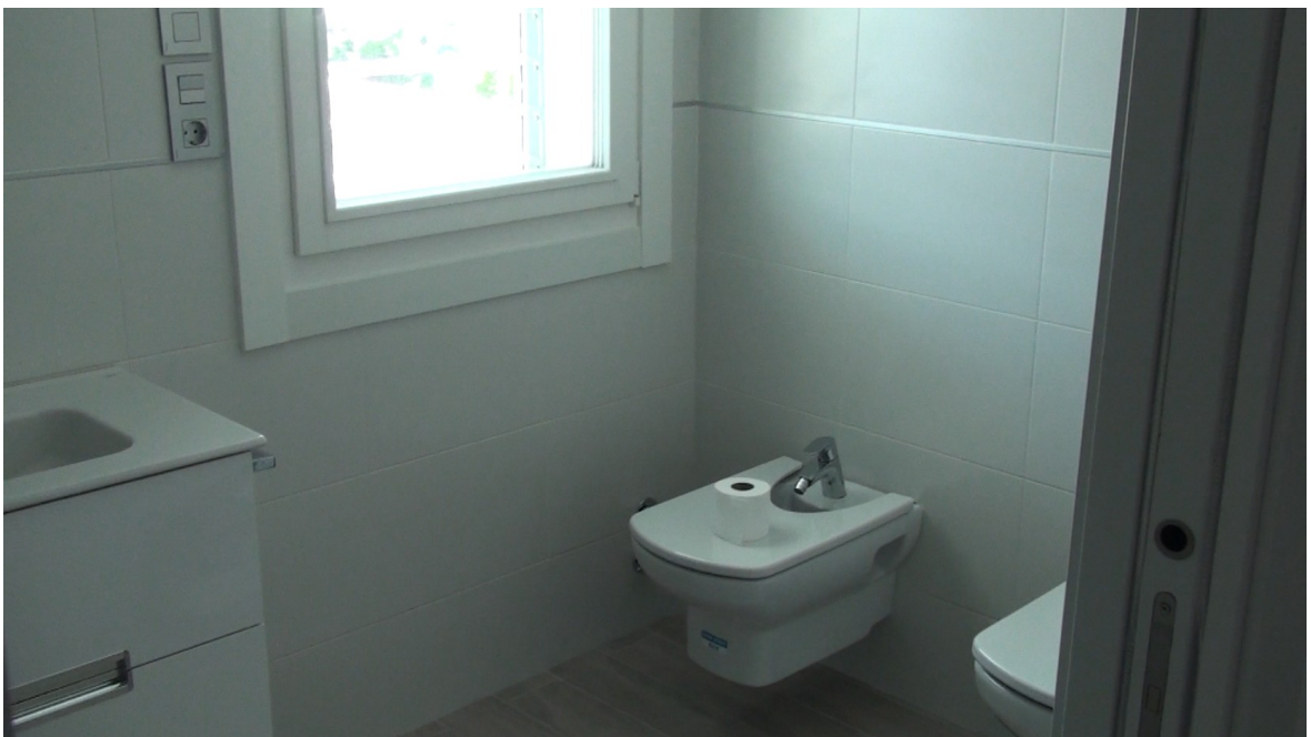
Toilets installed in the same bath as the previous photo
