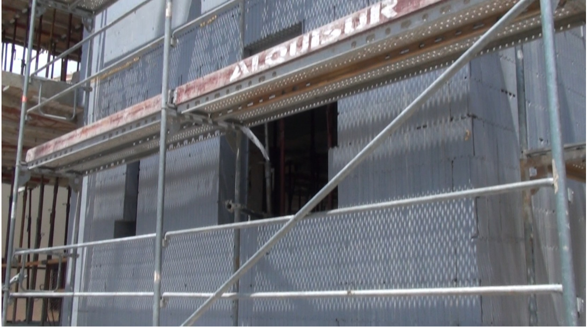
The following days – Perimetral scaffolding for safety reasons in the next storey
