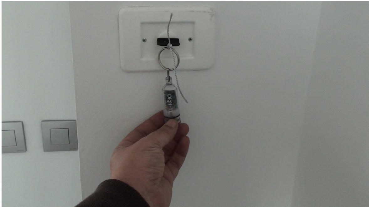
Detail of thermometer LabJack Digit-TL installed on the top floor of the house
