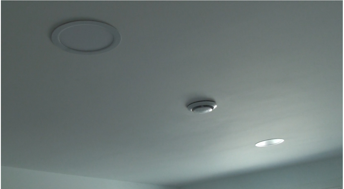
Mouth air insufflation renovated with two LED low energy lighting
