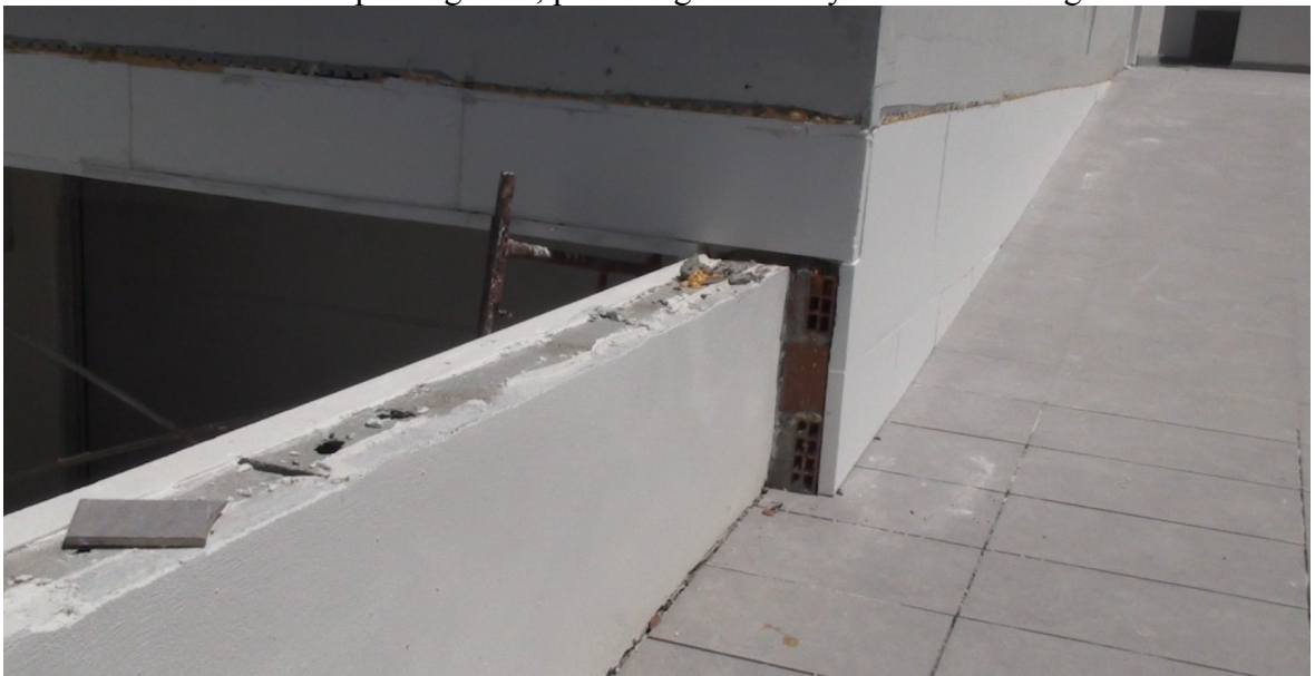
Insulation boards in front of the floor and the laterals not covered by soil
