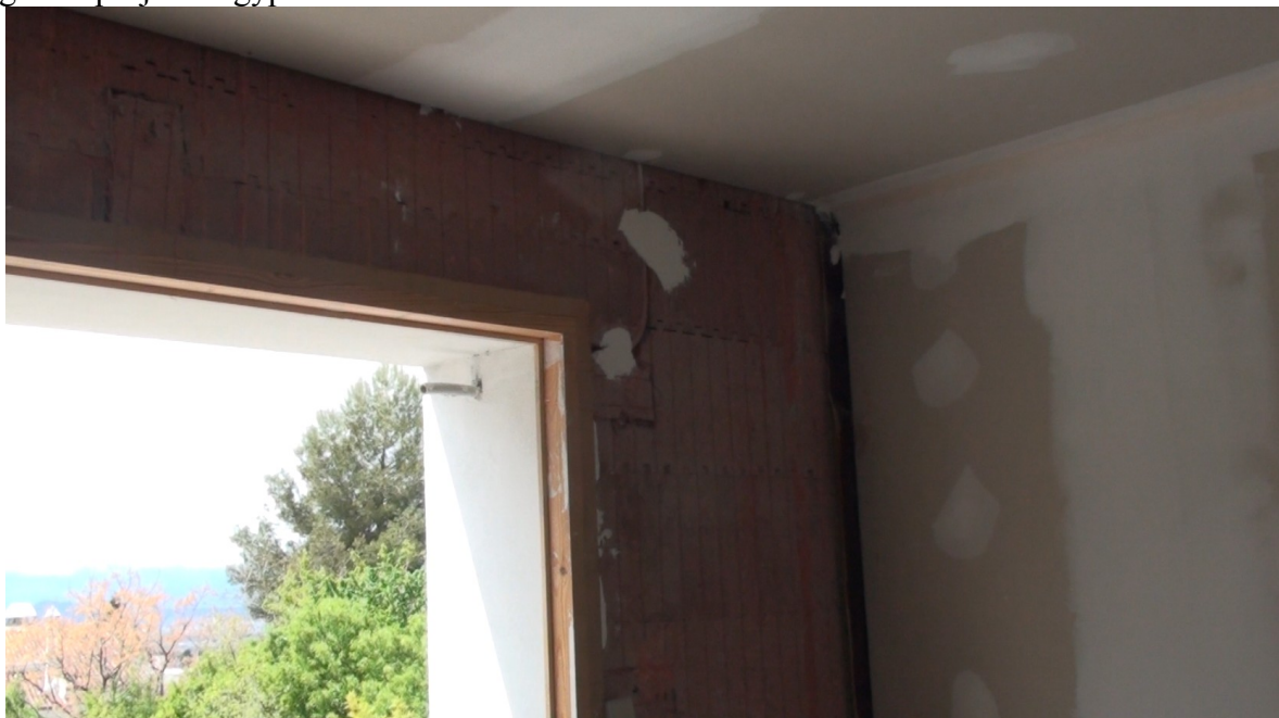
Rosy colour of insulation after application of means of adherence for the gypsum
