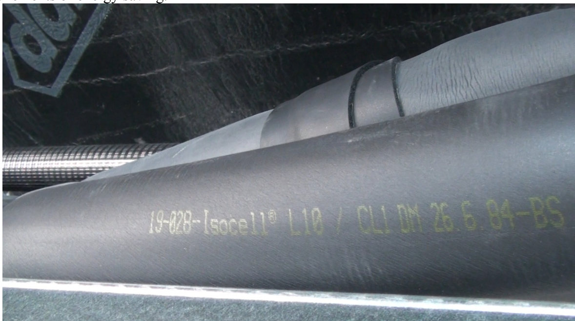
Thermally insulated by means of covering in an insulating shell all the tubes
