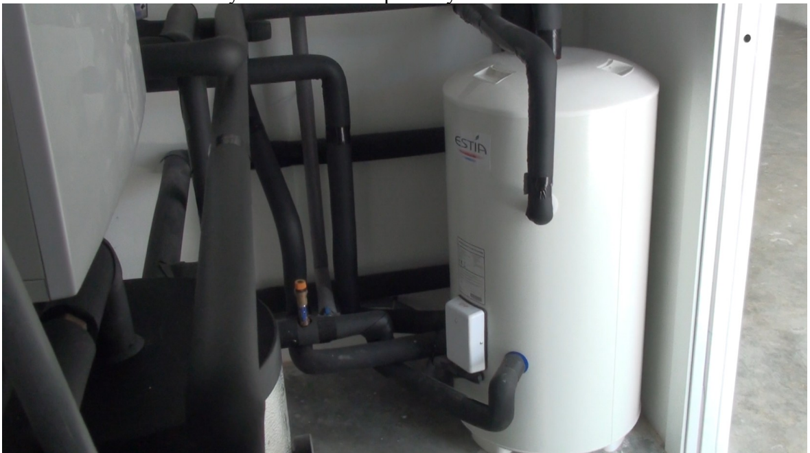
Deposit of ACS (warm sanitary water) with connection to the recirculation
