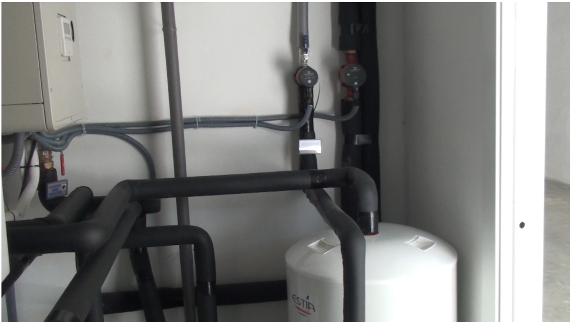
Above to the right, pumps for recirculation of ACS and impulse for floor heating
