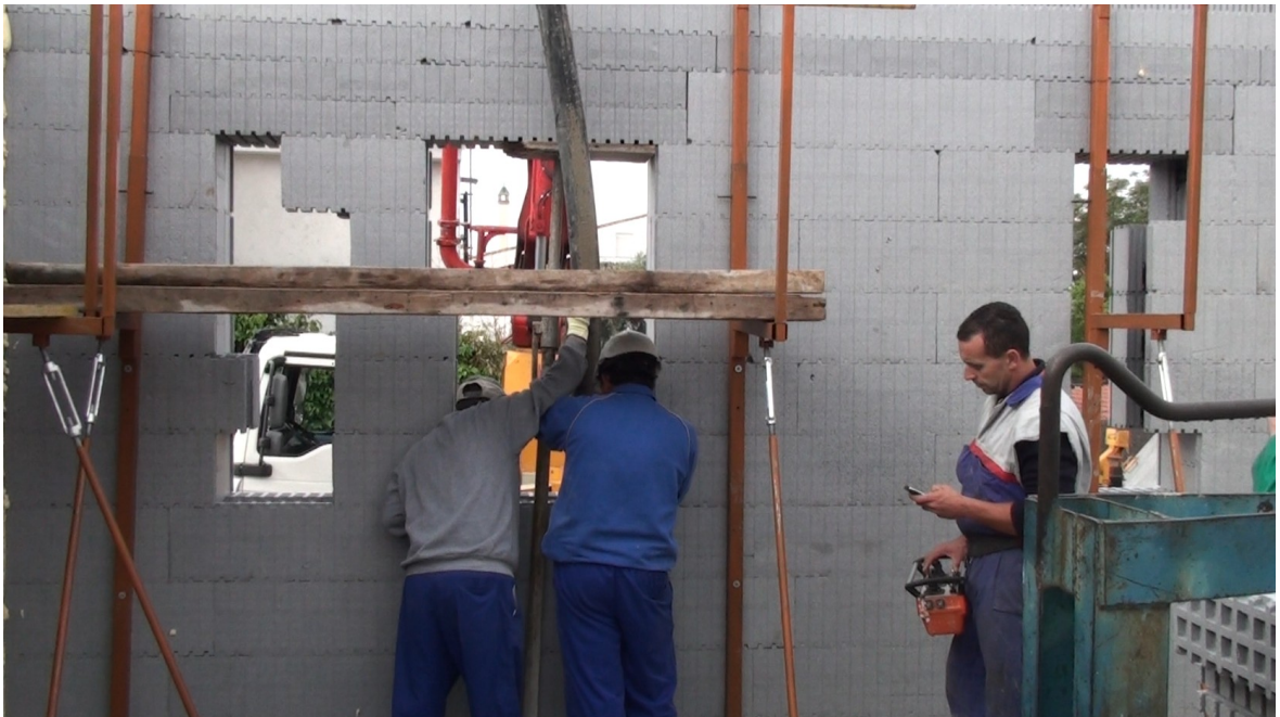
Day 3 25.04.14 – Pouring of concrete in a lower zone, from the window sill
