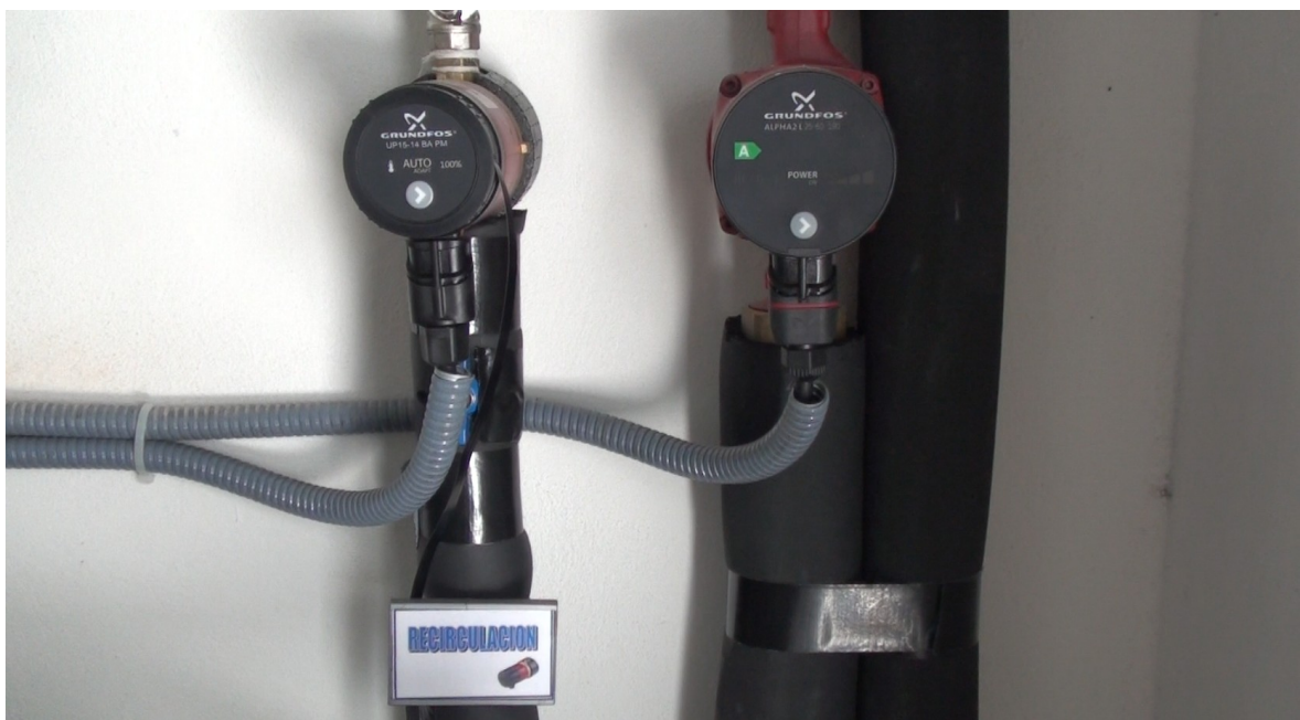
High efficiency pumps for the provision of the floor heating and the consumable water
