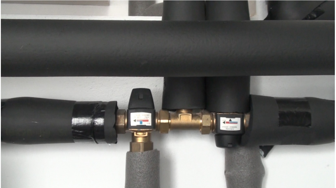
Thermostatic mixing and selecting valves to direct to consumption or the water tanks for ACS
