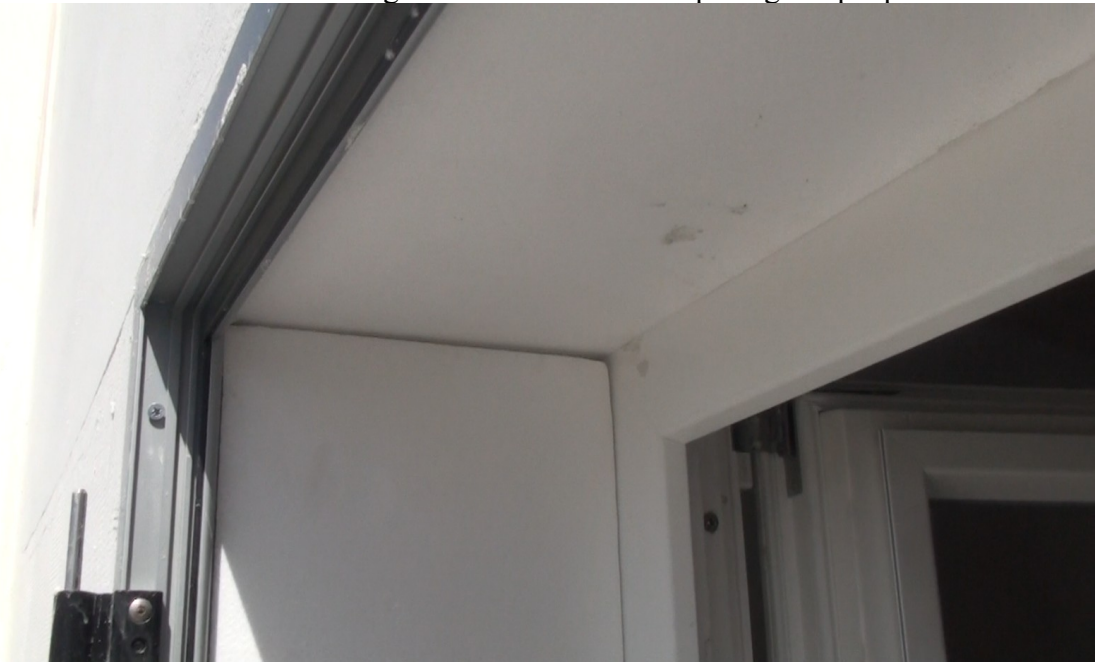
Example of an extra insulation board to cover part of the frame in the lintel
