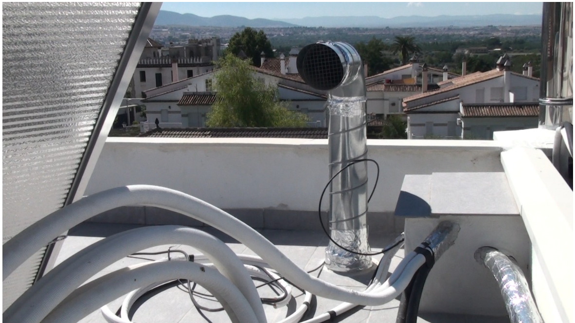
Exhaust tube for stale air on the upper roof
