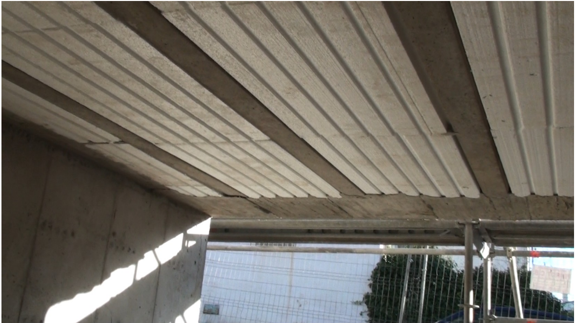
Insulating floor blocks in the floor of the ground floor (seen from ceiling of the basement)
