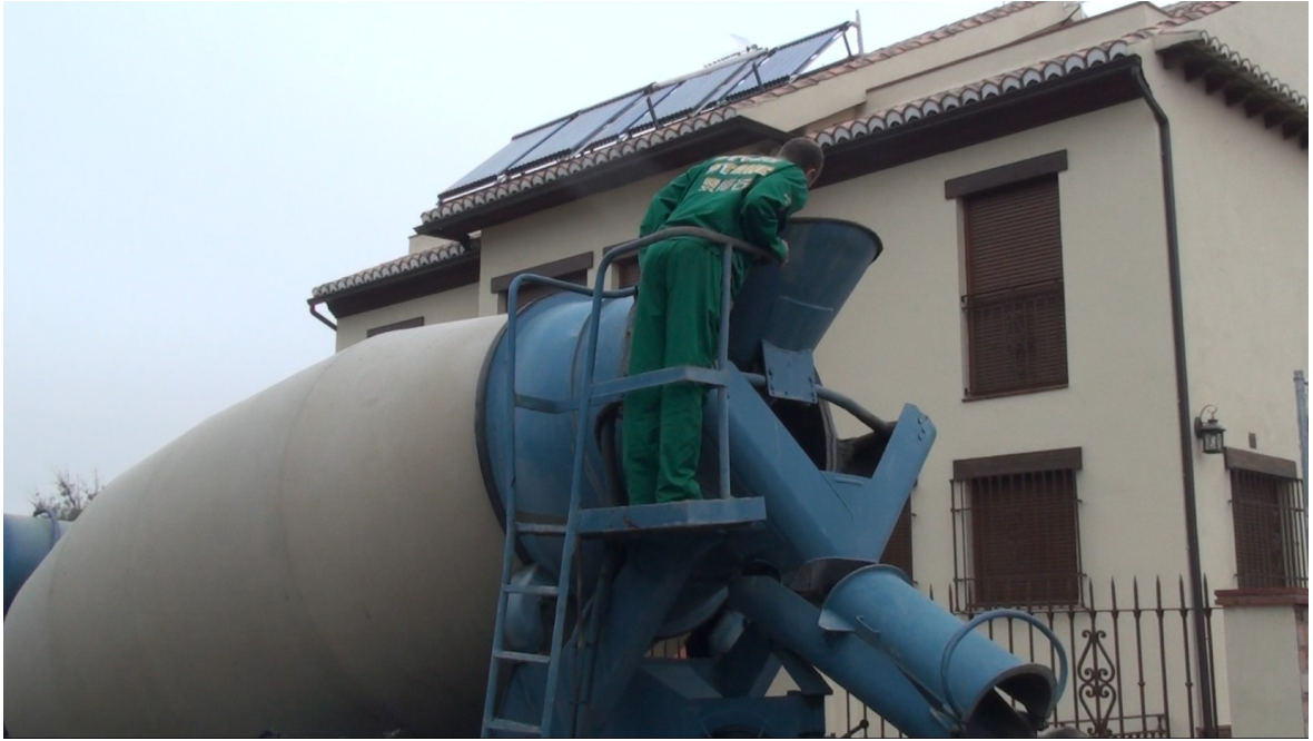
Day 3 25.04.211 – Checking the viscosity and gravel size of the concrete by Styro Stone
