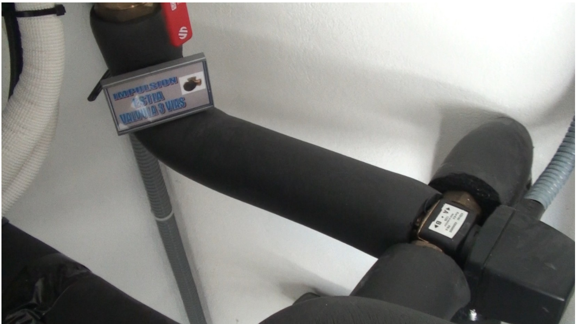
3-way valve selecting the circuit to warm in between ACS and floor heating.
