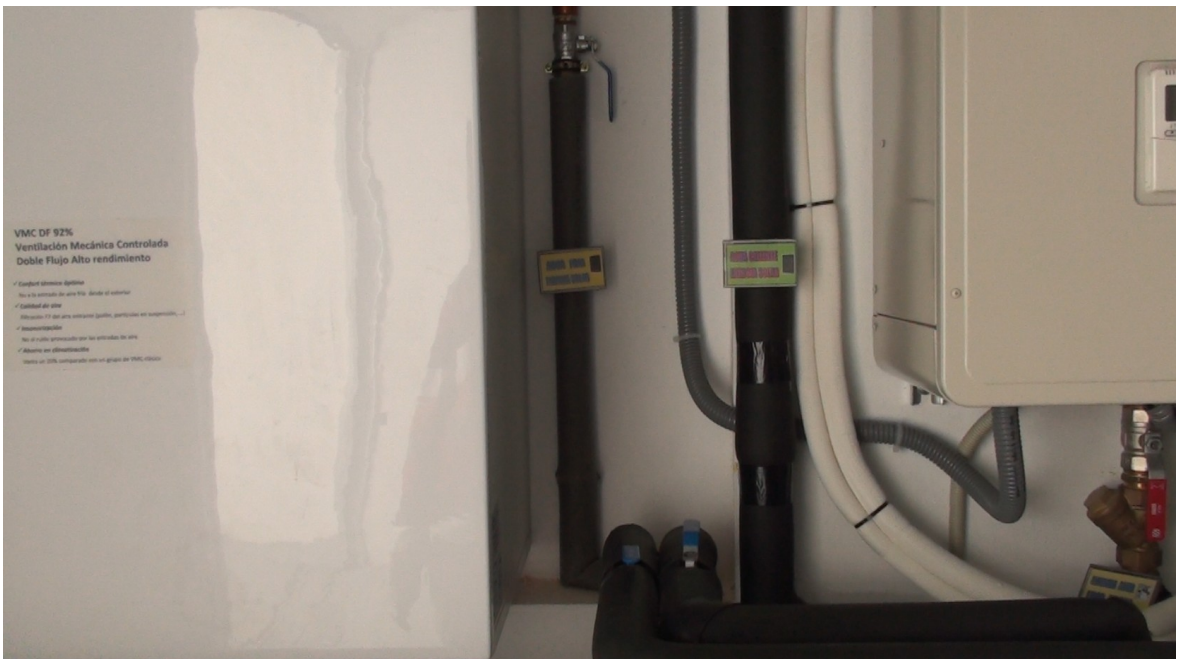
To and fro of water from the solar panels from the roof, insulated well
