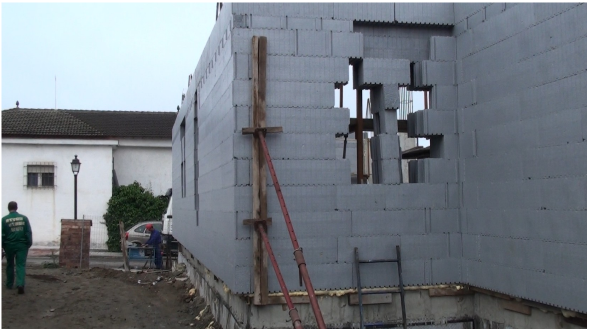
Day 2 20.04.2011 - Completion of the wall in full height with the help of Styro Stone
